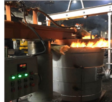
Fossil Fuel Fired Preheater ( HSD )Emission due to fuel burning, flexible, easy to use.
