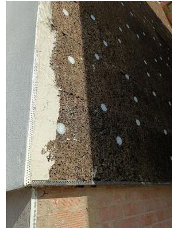
Cork insulation ( \lambda=0,040 W/mk) on the façade
